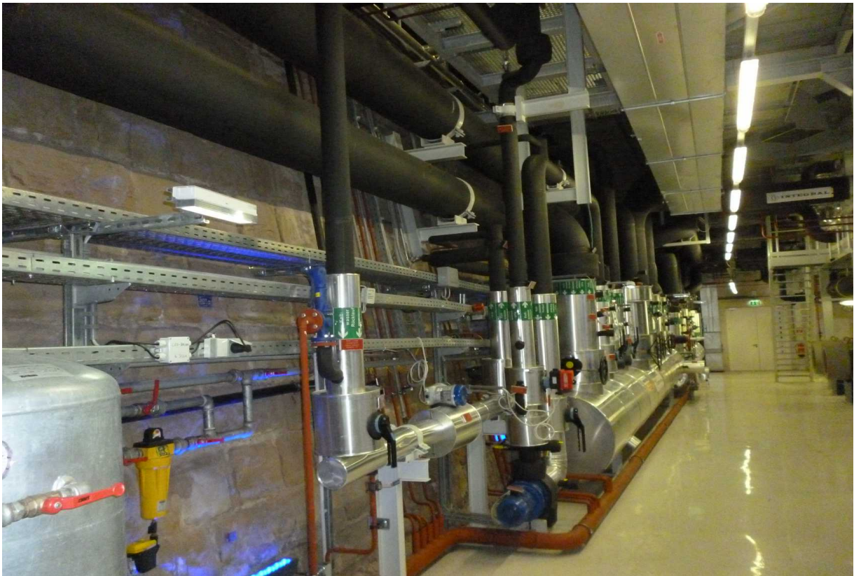
Picture 3. State of The Art District Heating & Cooling System of Spittelau WTE Plant
