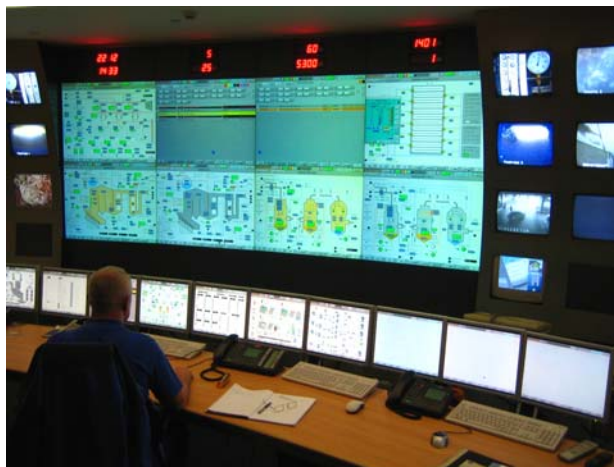
Figure 7: Control room of the WTE facility Spittelau
