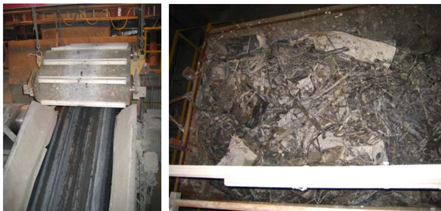
Figure 4: Left: Overhead electromagnets recover ferrous scrap from the bottom ash; Right: Recovered ferrous scrap
